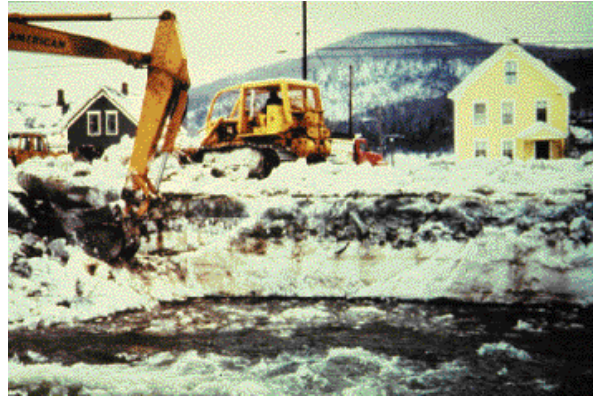
Figure 3-18. Breaching an ice jam in Hardwick, Vermont, using excavation equipment working from the shore and a bridge (bridge is not shown, but is just beyond the left edge of the photograph).
