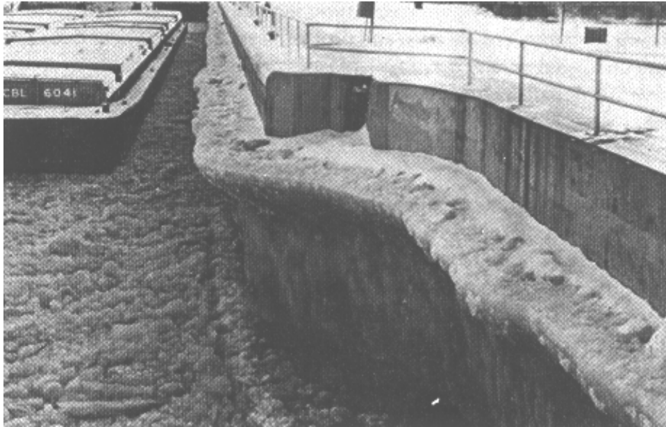
Figure 14-4. Ice collar formation on the gate recess and chamber walls, restricting the full opening of the miter gates and limiting the usable width of the lock
