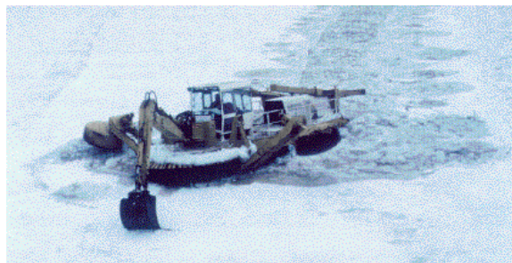
Figure 3-11. Breaking ice with an amphibious excavator on the Aroostook River, Ft. Fairfield, Maine.
