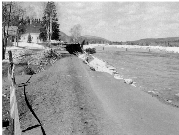
Figure 10-8. Bank scour caused by a breakup jam near Dickey, Maine.
